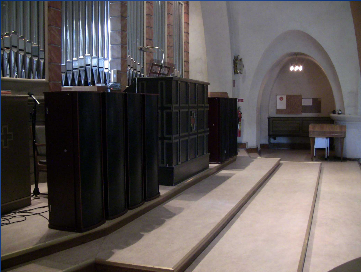
Particulate air cleaning: Eight stand-alone air cleaners assembled on the balcony of a church. Measurements have indicated effective reduction of the amount of airborne particles.
