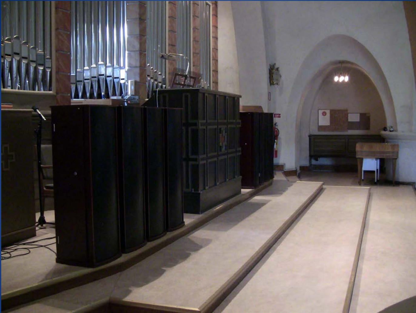
Particulate air cleaning: Eight stand-alone air cleaners assembled on the balcony of a church. Measurements have indicated effective reduction of the amount of airborne particles.
